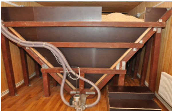
Figure 19. Pellet boiler fed by a 9-ton reserve. We can see the suction motor at the base of the silo. This model is also equipped with a worm screw
